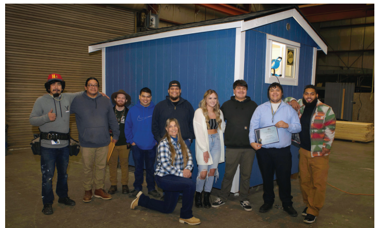
Pre-Apprenticeship students in the Tulalip Tribes TERO Vocational Training Center building a tiny house for homeless people. Materials for each tiny house cost $4,200. State program provides funding through ANEW.
